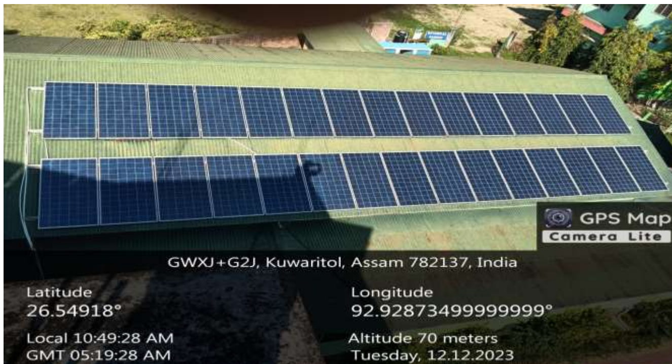
Hybrid Solar Power Plant of 40KW
