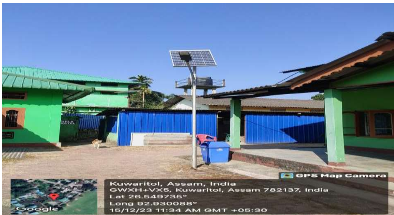
SOLAR STREET LIGHT AT COLLEGE CAMPUS
