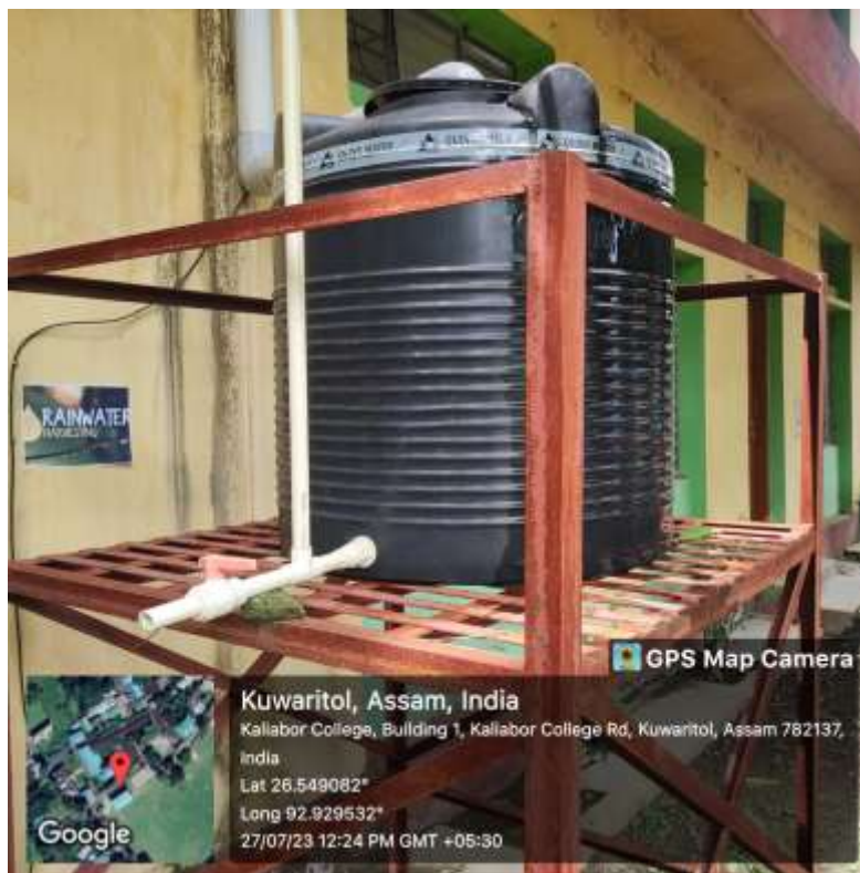
RAIN WATER HARVESTING
