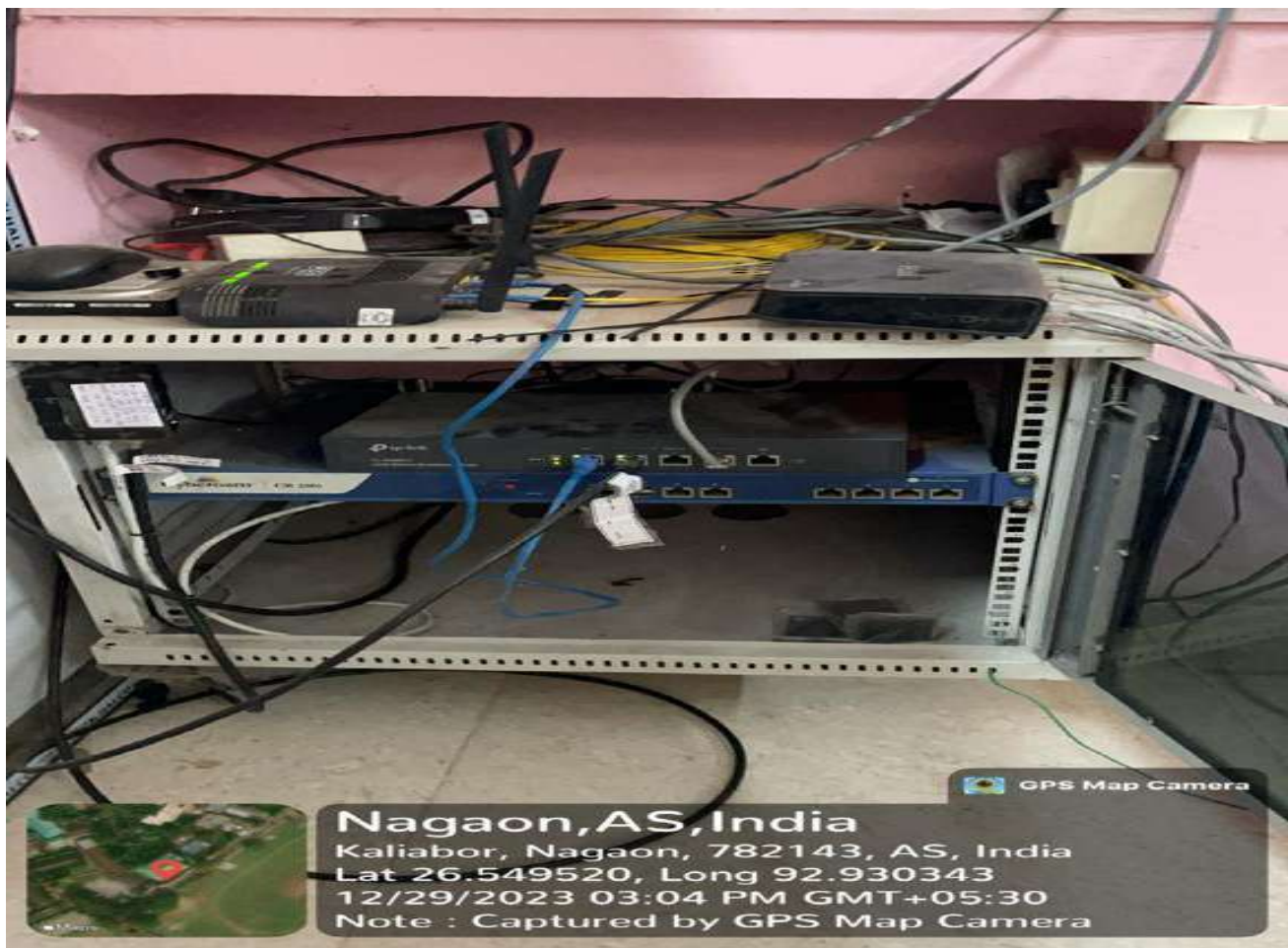
ROUTERS AND SWITCH
